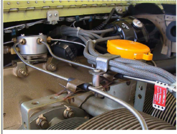
D) Installation of RPM sensor, overview
